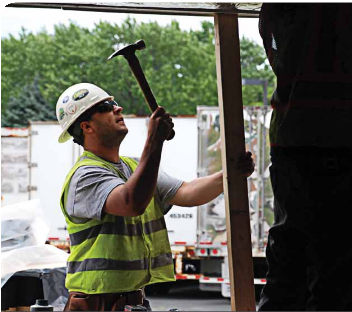
Washburn's flexible learning space was created during construction this summer, which included safety enhancements approved by voters in the 2013 referendum and a comprehensive school maintenance project.
